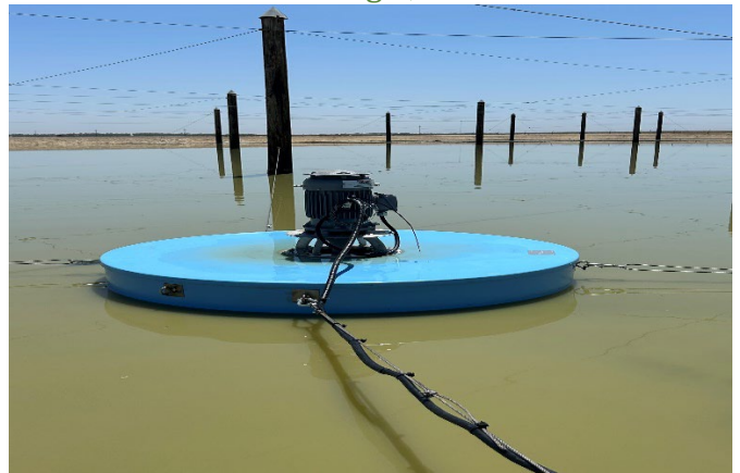
Image of the New Aerator Installed Aug 5, 2026
