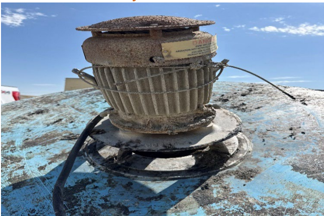
Image of the old Aerator More than 15 years old
